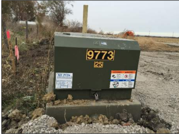
Photo #19 Pad-mounted transformer, located on the south side of the Property.
