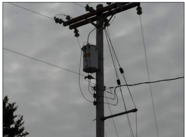
Photo #18 Pole-mounted transformer, located on the west side of the Property.
