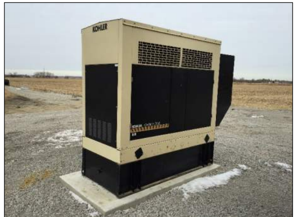
Photo #16 Generator, located on the south side of the Property.
