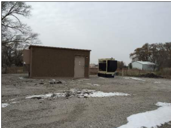
Photo #15 Utility building and generator, located on the south side of the Property.
